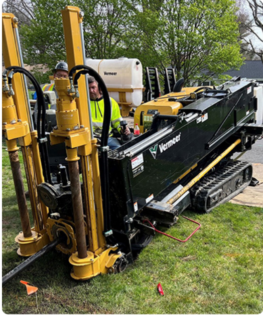
Custom Underground employee operates horizontal directional drilling equipment during fiber optic installation.
